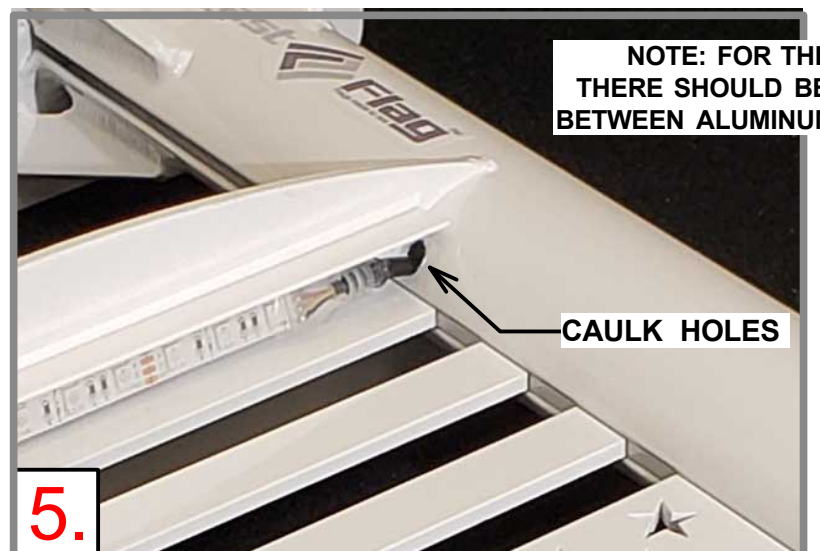
ONCE LED STRIPS ARE ATTACHED TO DEFLECTOR, THEN SILICONE THE ALUMINUM DEFLECTOR SHIELD TO THE FLAG AS SHOWN. CAULK ACCESS HOLES ONCE POSITIONED CORRECTLY TO PREVENT WATER INTRUSION.
